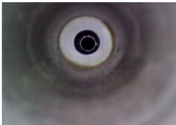
LC3 - Oxidation detected after 14 cm of insertion.
