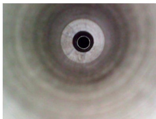
LC8 - Oxidation and grooves detected after 13 cm of insertion.
